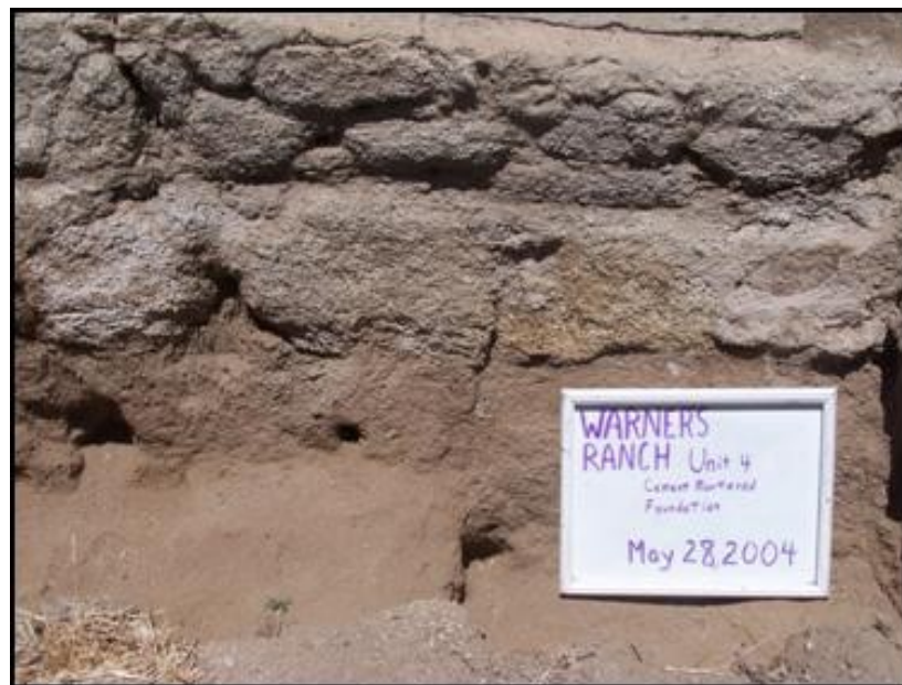
Figure 10.15. Cement mortared facing at the base of the Warner's Ranch House east wall in Unit 4. Courtesy Stephen R. Van Wormer and Susan D. Walter.
