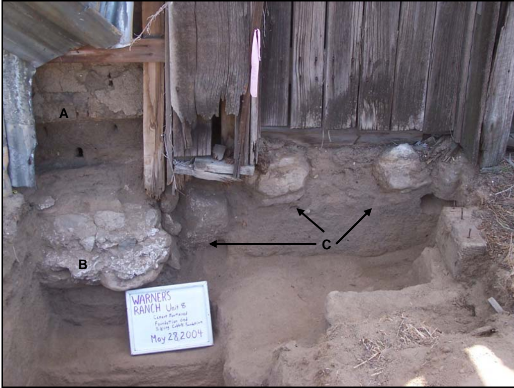
Figure 10.30. Unit 8, showing the adobe blocks of the western wall of the center wing (A), lime mortared cobble facing on the foundation of the center wing (B), and the remains of the cobble foundation for the original adobe wall on the west side of the south wing (C). Courtesy Stephen R. Van Wormer and Susan D. Walter.
