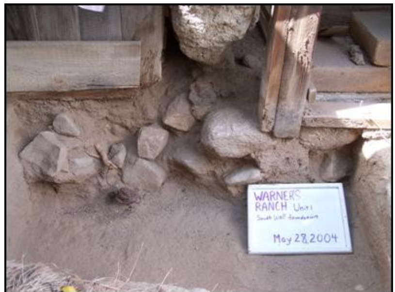
Figure 10.8. Cobble foundation in Unit 1. The west half is badly disturbed while the eastern portion remains intact. Courtesy Stephen R. Van Wormer and Susan D. Walter.
