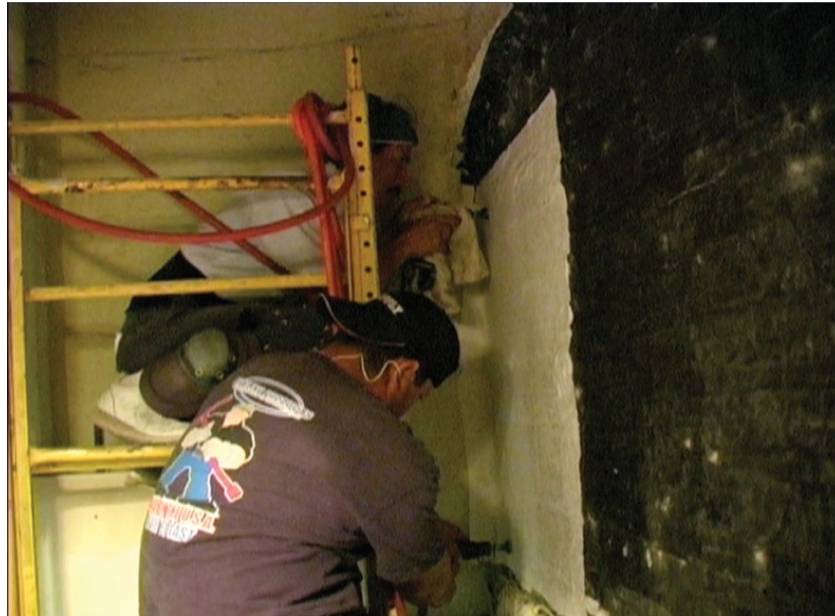
Figure 5.17. The fabric is sealed with black electrical tape. Courtesy of Seth Mallios and Donna Byczkiewicz.
