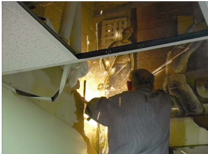
Figure 5.8. Nathan Zakheim cuts part of the lowered ceiling frame in order to gain access to the base of the mural. Courtesy of Seth Mallios and Donna Byczkiewicz.
